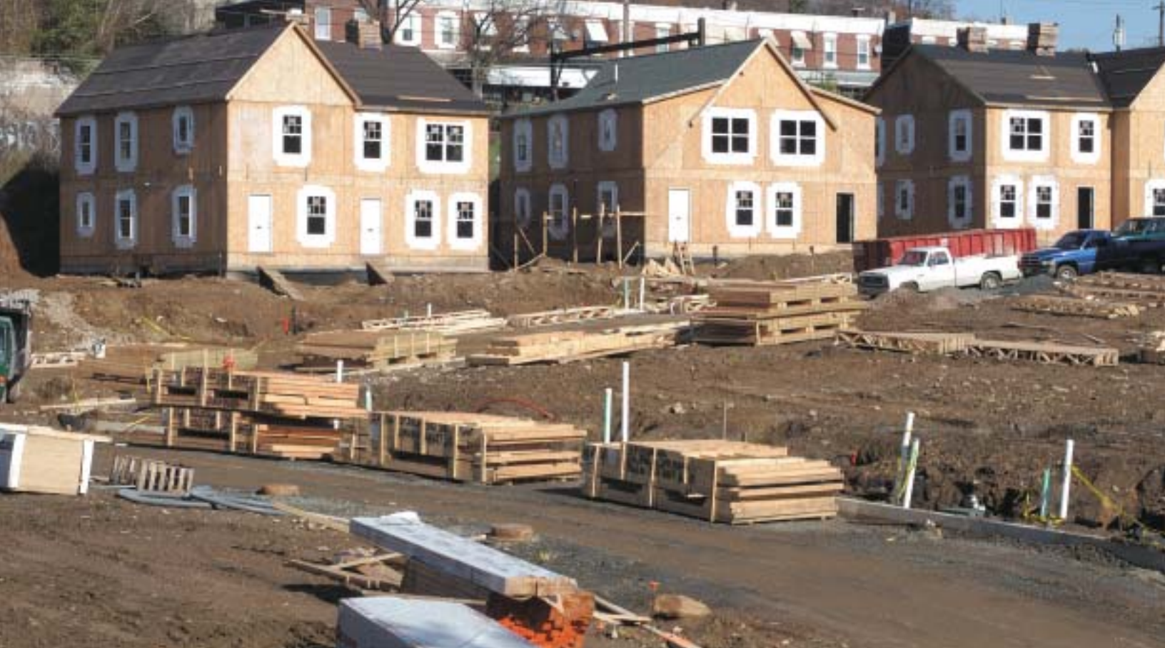
PHA's innovative financing techniques have accelerated the pace of new construction in Philadelphia.
